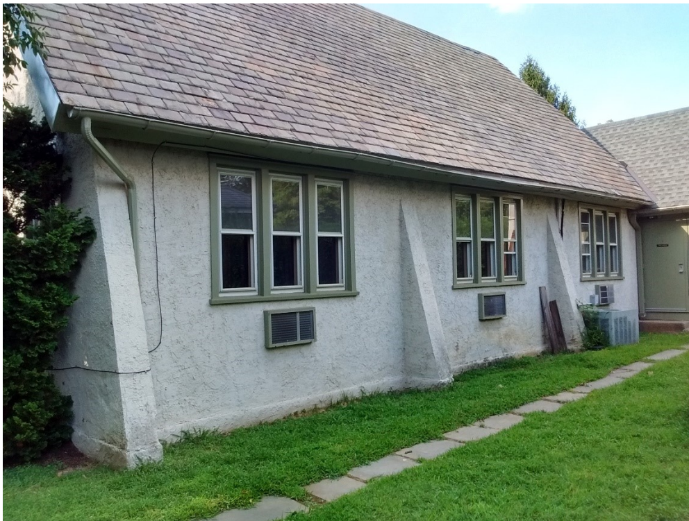
Figure 11: South side of chapel showing grouped windows and plain, angled buttresses. Steven Peitzman, August 2019.
