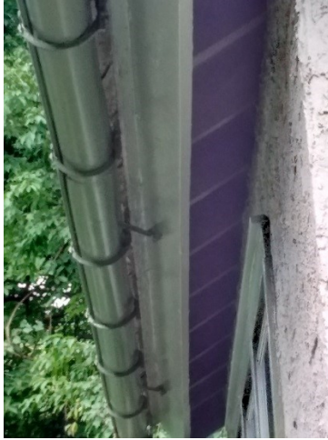
Figure 10: Exposed rafters in unenclosed eave, north side of chapel. Steven Peitzman, August 2019.
