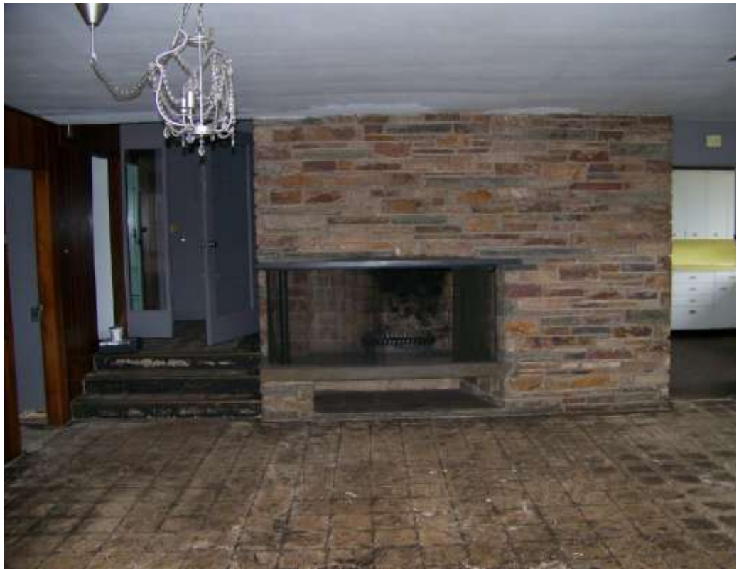
1951 Stone fireplace with slate mantle, vinyl asbestos tile has been removed, yellow laminate counter and backsplash and white metal Geneva cabinets are visible at Kitchen
