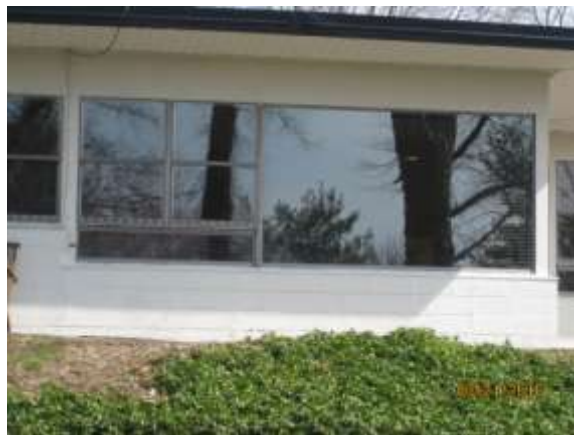
1951- Cupples single pane windows with storm windows Cupples double pane windows Masonite panels run continuous above windows
