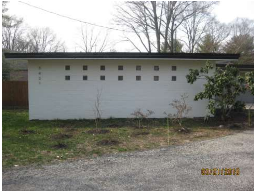
2009- East Elevation- In 2009, an 18' translucent corrugated fiberglass overhead garage door was removed and was infilled with in-kind materials
