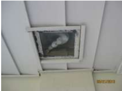
1974- Similar Downlight used at Exterior Garage Addition
