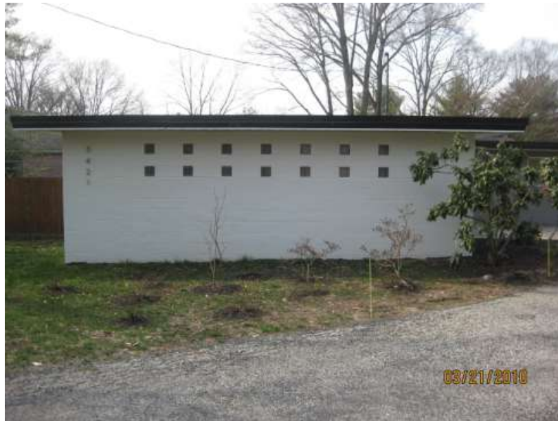
2009- infill at garage using parged, scored cinder block and Pittsburgh Corning Glass Block
